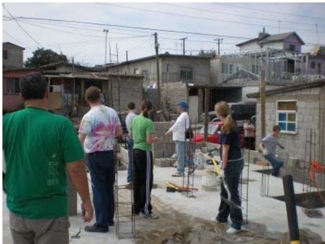
AHS Student Rachael Breaux (with shovel) helps work on the foundation for a home in Ensenada, Mexico
